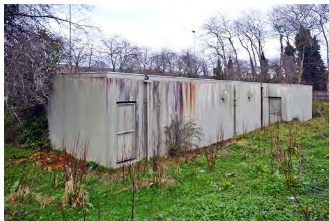
Stormont's 1950s Sub Control understood to have been sealed since 2011. Photo Chris Rayner
